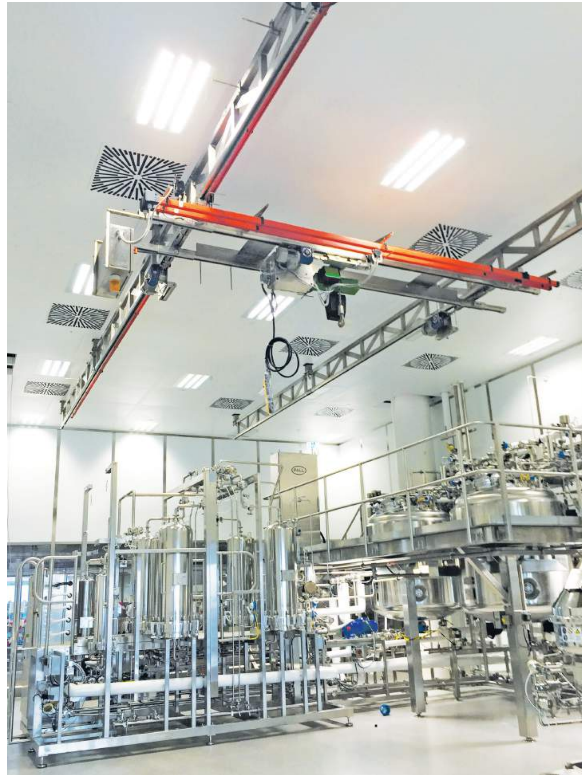
Completely motorized overhead stainless steel cranes with upraised double girders and support for conductor bars in pharmaceutical industry.
