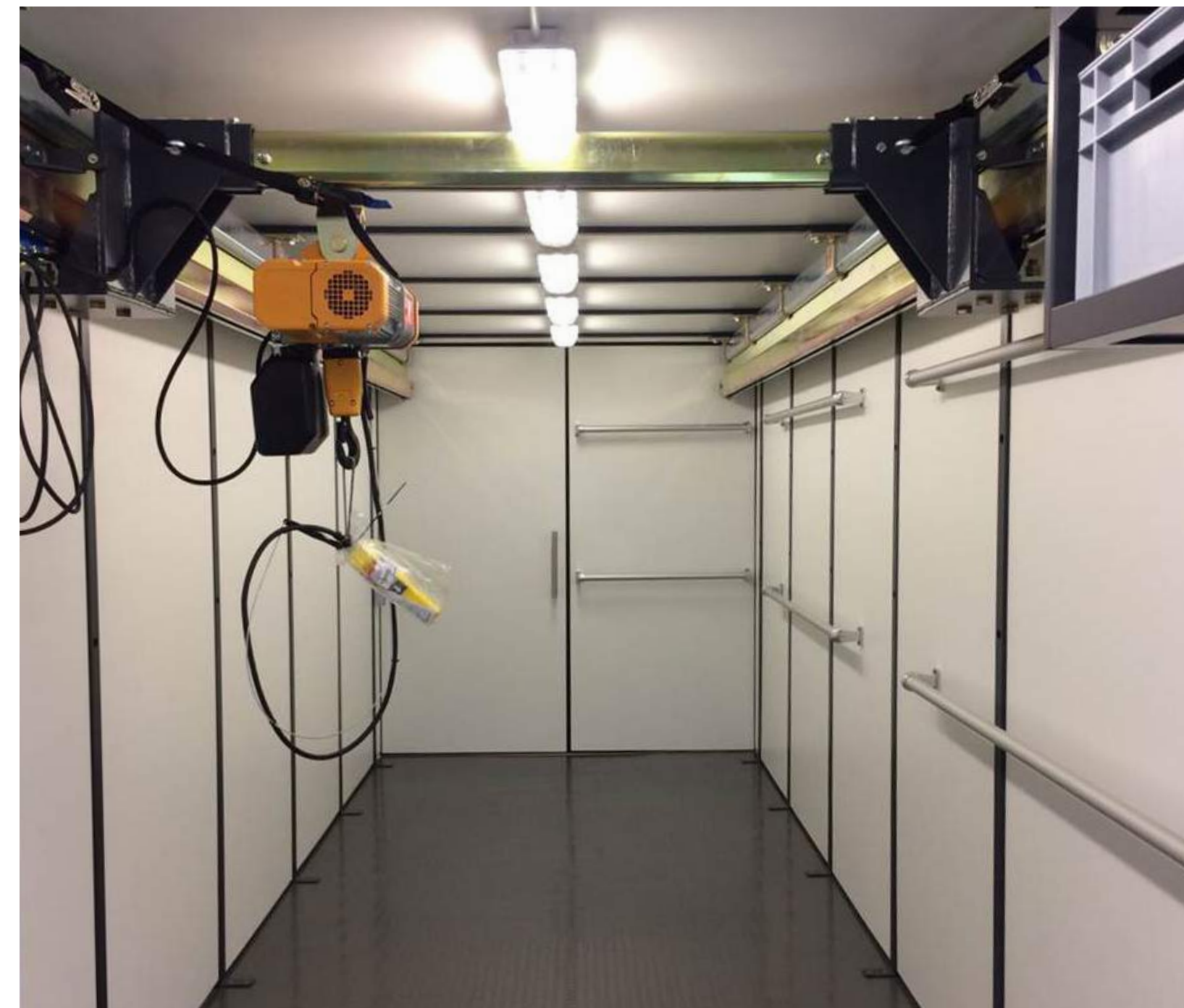
Light crane system installed inside a container
