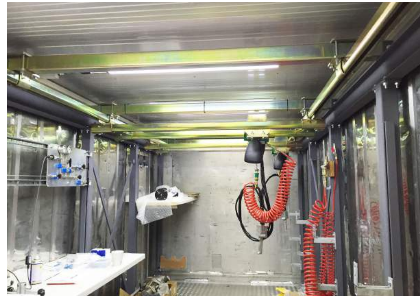
Low headroom light crane in constrained space room.
