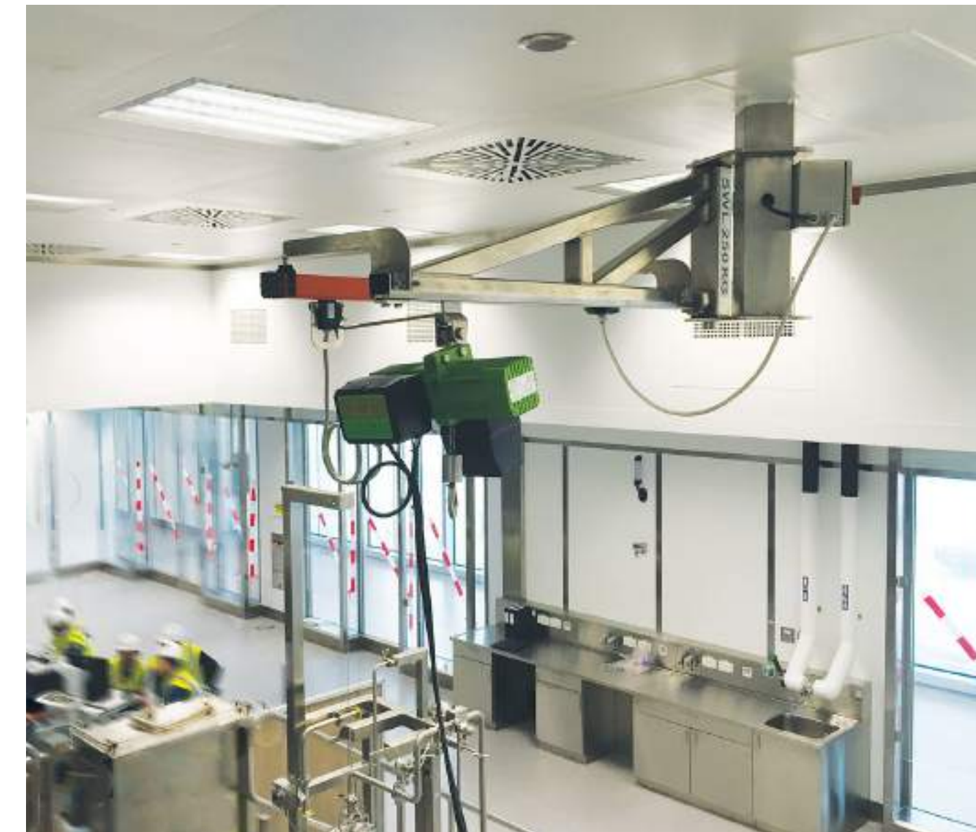
Stainless steel jib crane mounted on the ceiling.
