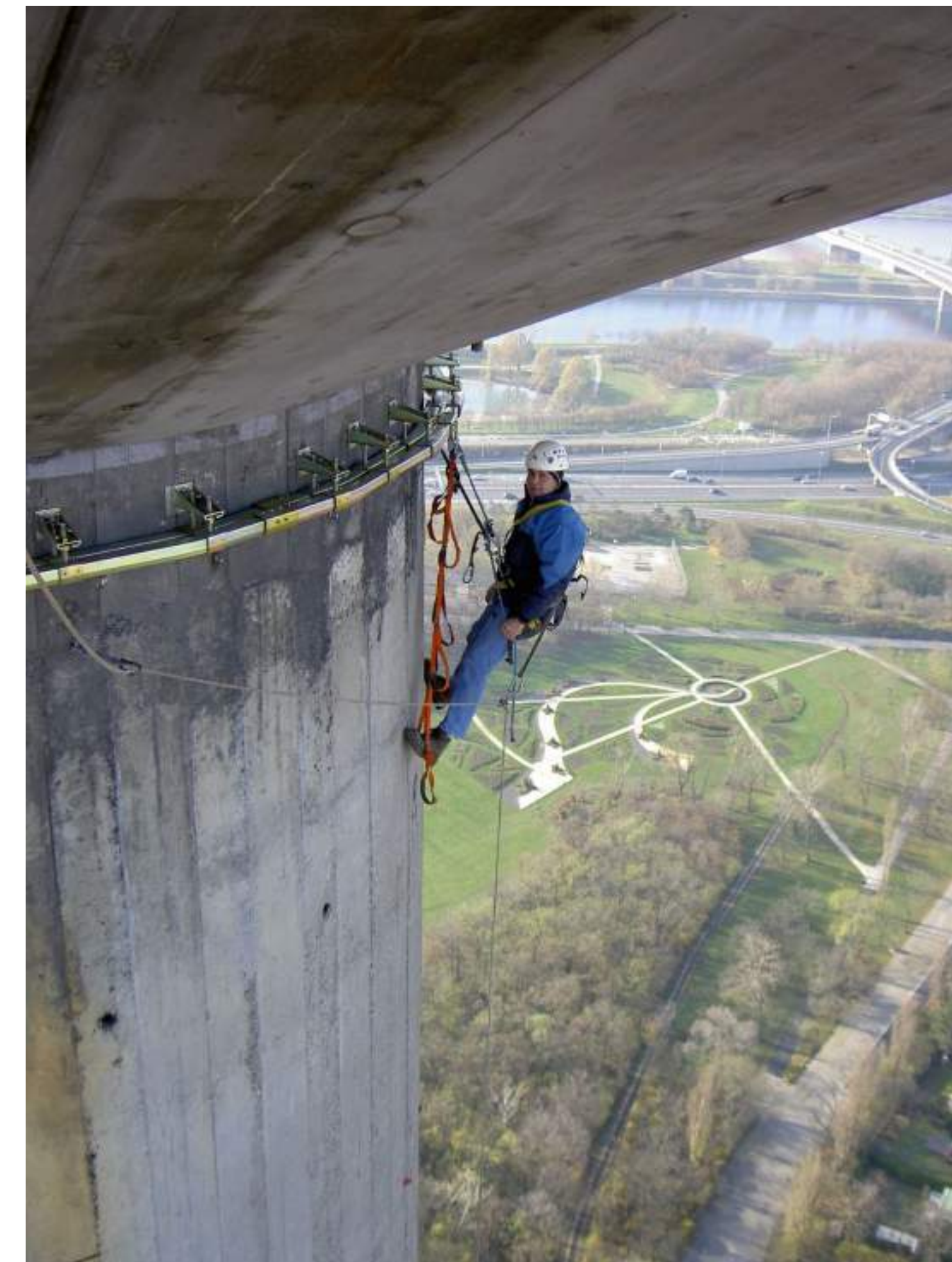
Inspection processes in the Danube tower in Vienna. The system was mounted around the building with special support brackets to allow for the free movement all over the working area.
