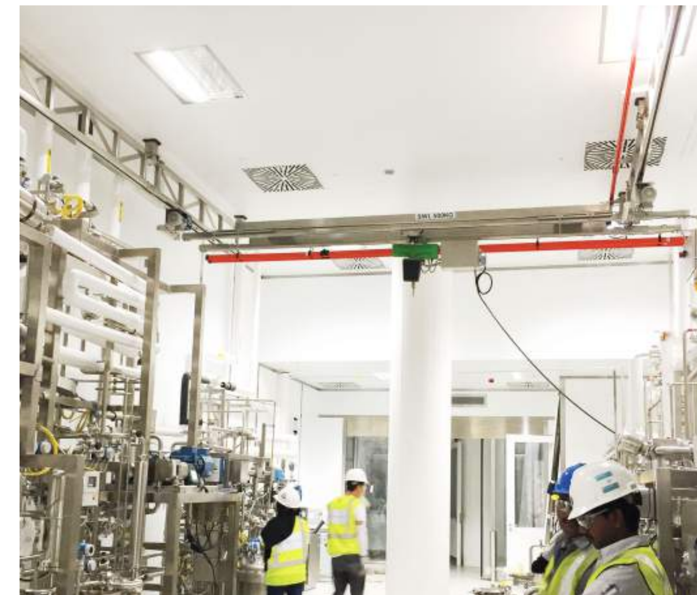
The trussed/reinforced runway tracks were mounted on steel beams of the existing building construction, at the maximum height possible.
